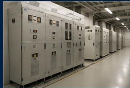
POWER FEED EQUIPMENT (PFE)
